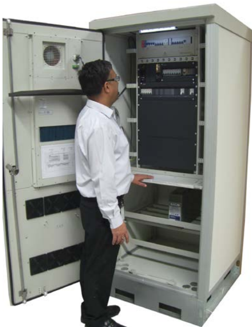
Enclosure Internal View
